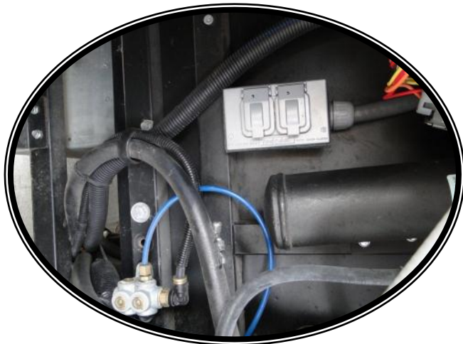
Weatherproof Plug on Firewall
